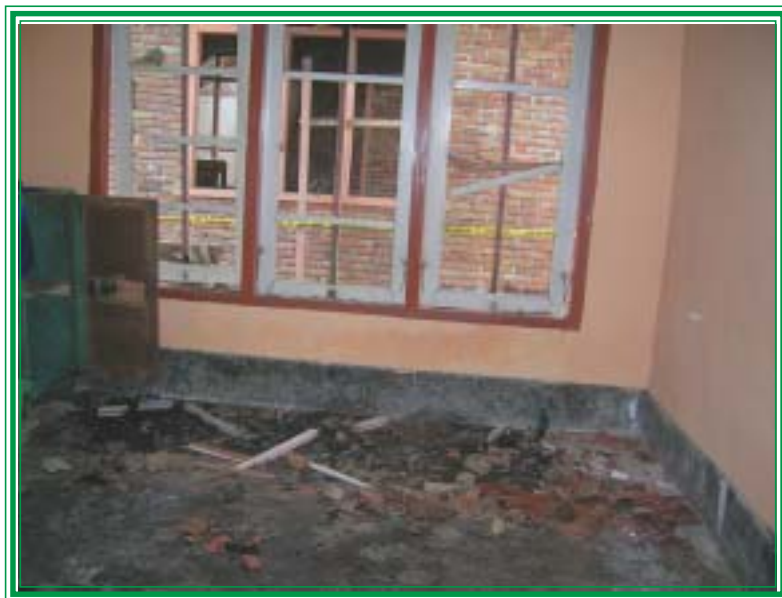
► Location of a house of member of the Ahmadiyah which was damaged in the attack in Loteng, West Lombok in March 2006.
